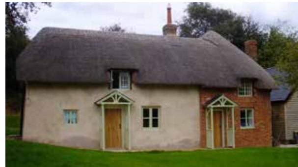
Sympathetically restored cottage with cast iron windows, timber porch and windows remade to match the originals.
