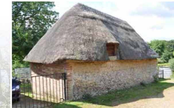
Building of local interest - outbuilding with flint and cob wall under a thatched roof at Godshill.
