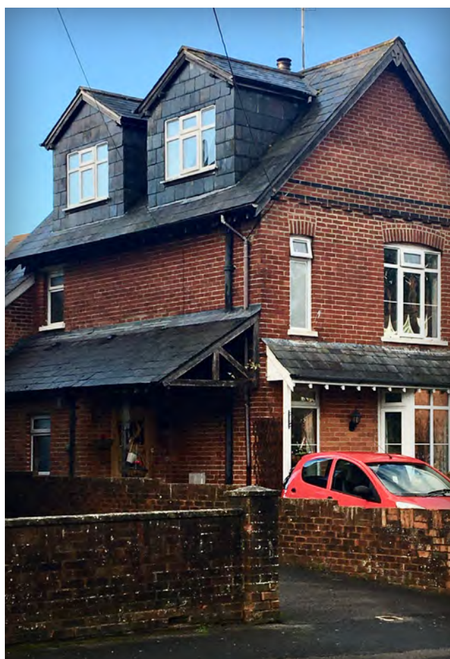
The large dormers feature wide cheeks, which appear heavy and out of proportion with the scale of the cottage
