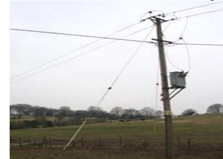
Overhead wires Blissford
