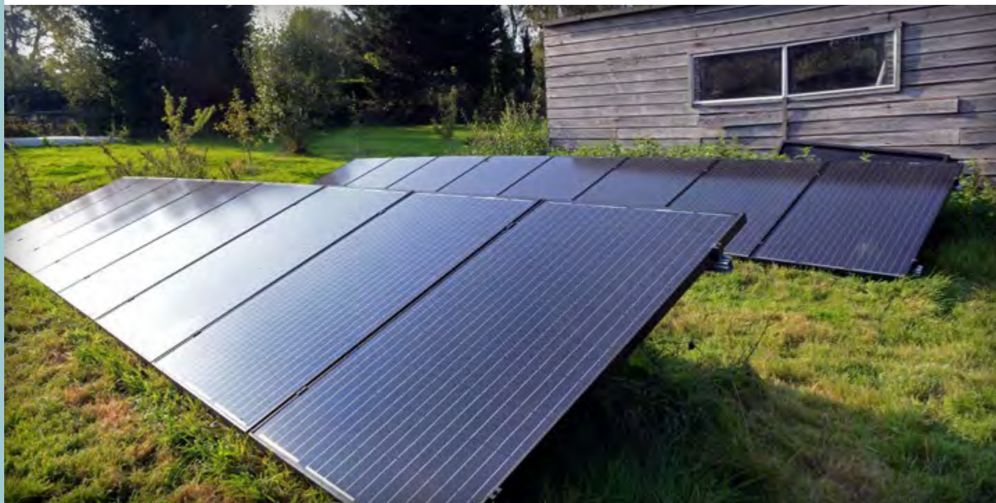
Ground mounted solar panels at Efford Mill
