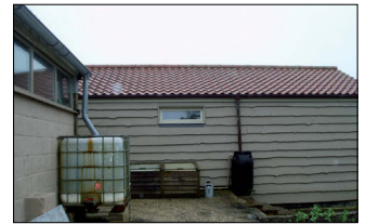
Opportunity to recycle water direct from roof
