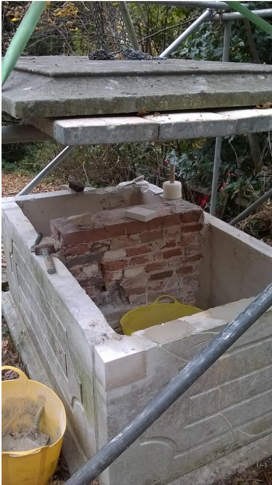
Work in progress to a listed tomb at St Michael's churchyard in Lyndhurst
